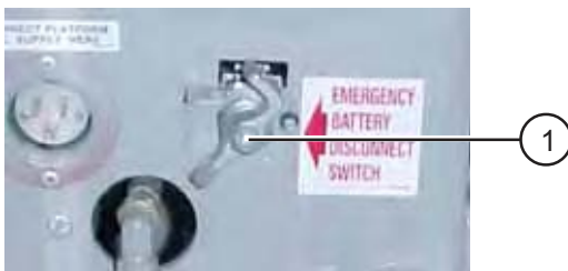
Figure 2-5. Emergency Main Power Disconnect Switch
