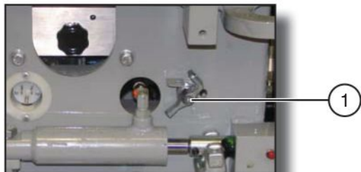
Figure 2-1. Main Power Disconnect Switch
