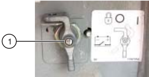
Figure 2-1. Main Power Disconnect Switch
